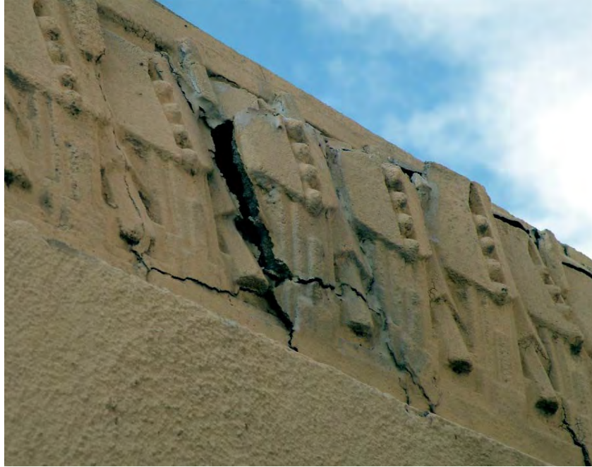
#8 – Typical Decorative Cast Stone Damage
