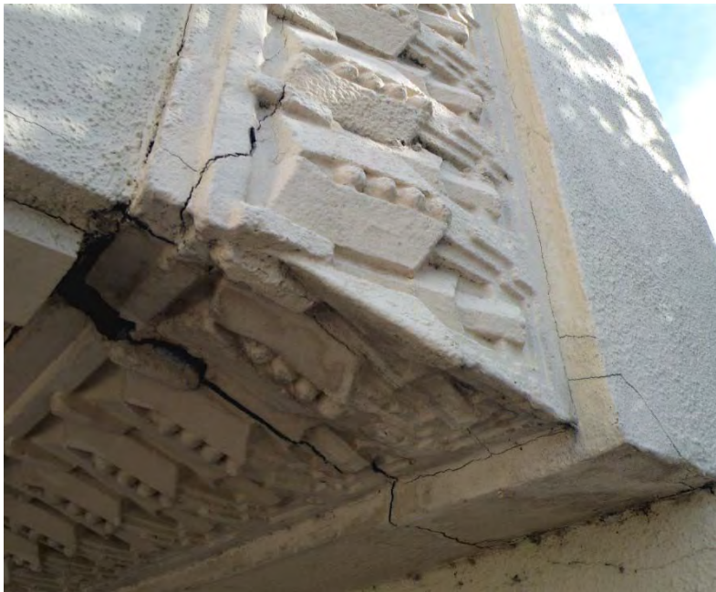
#7 – Damaged Decorative Cast Stone at Balcony
