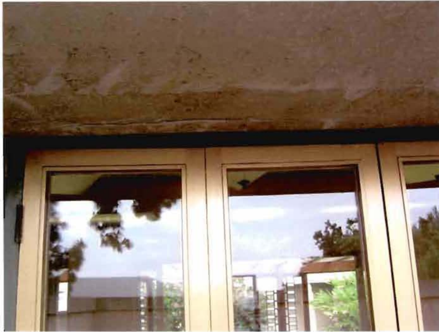
PHOTO 17 - Gallery Exterior Ceiling Above Door Entrance at Line B/4.8
