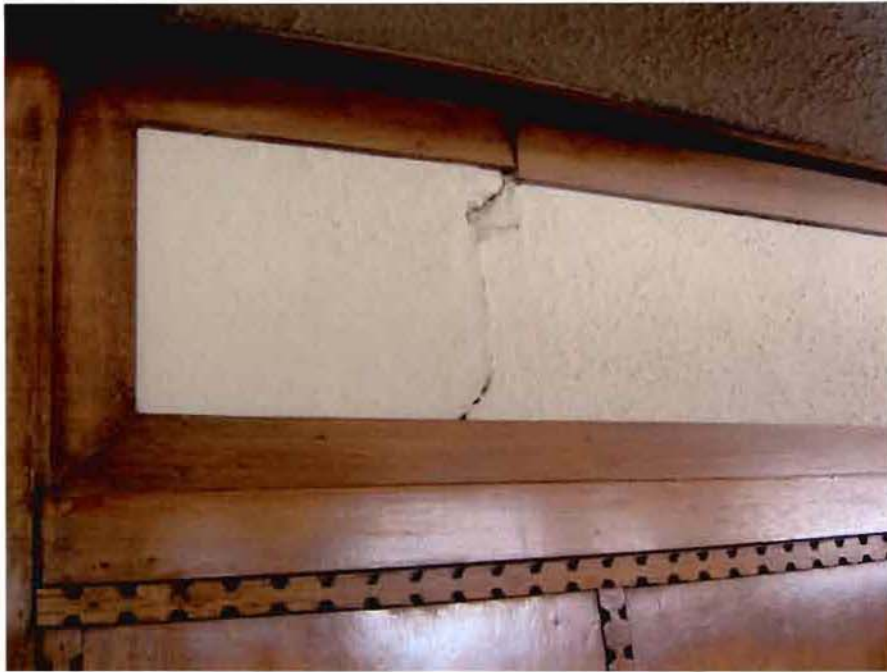
PHOTO 5 - Dining Room Interior Walls at Line F/6.2
